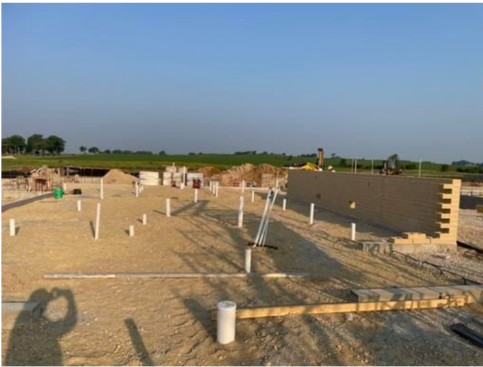
Masonry being installed on Bath House Taken on Jun 23, 2023, 7:12 AM CDT Added on Jun 23, 2023, 8:30 AM CDT Added by andrew gordon
